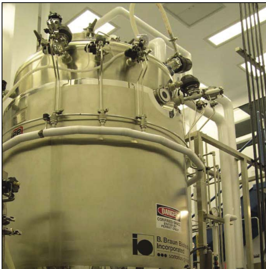
Figure 5. Front view of the 2,500L bioreactor: This 2,500L bioreactor was designed more vertically than horizontally to take advantage of the 25-foot high bay ceiling space. Most utility piping was routed above the facility and down to process equipment, thus reducing much of gray space otherwise needed for utility piping at the ground level.
