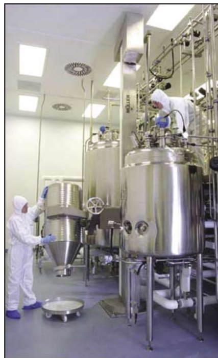
Figure 2. GMP Media Make-up Suite with GMP Manufacturing Facility.
