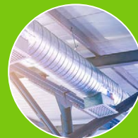
HVAC Systems & Classified Areas
